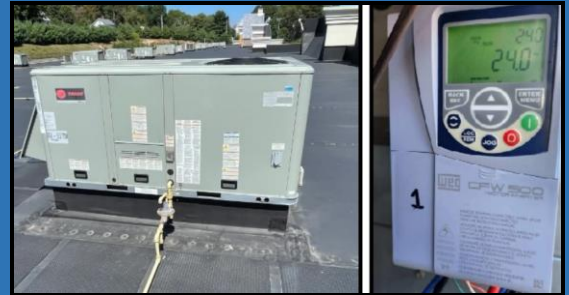
A Roof-Top Unit with Advanced Rooftop Controls
