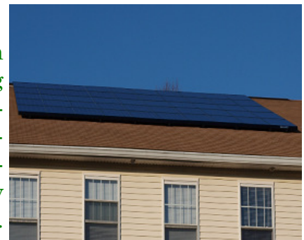
Solar panels doing their magic
